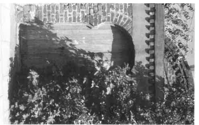
Figure 5. Derelict baths Note brickwork where plaster has fallen
